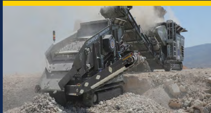
The crushing machine and screen have started recycling the rubble generated by the earthquake.
