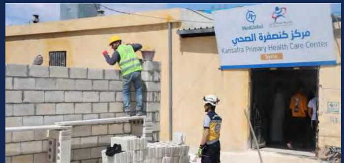
Rehabilitation of 15 health centers (hospitals and primary care centers) damaged by the earthquake.
