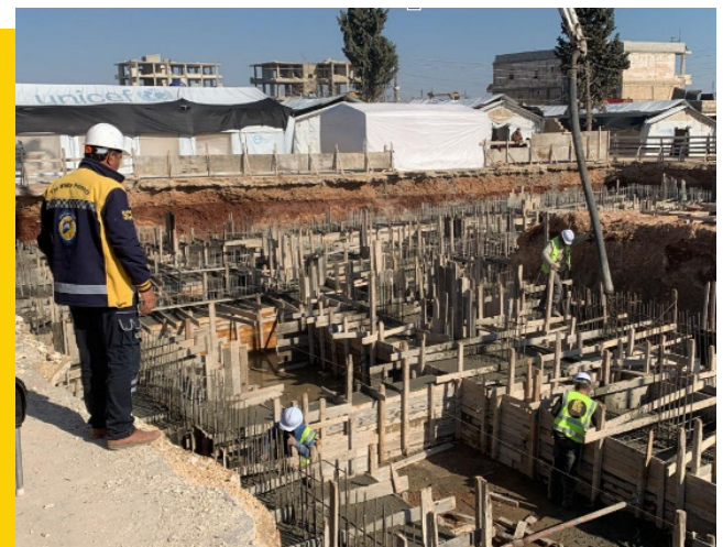
Construction of the Khalid bin Al-Walid School in Jandairis, pouring a reinforced concrete foundation.
