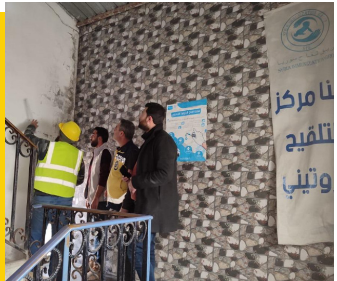
Rehabilitation of 15 health centers (hospitals and primary care centers) damaged by the earthquake.
