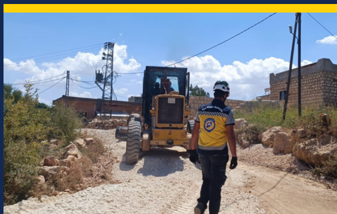
Rehabilitation of roads from Sijer - Bqesemtoh to Al Fidaa Camp and from Kafruhin to Bishmaroun Camp.
