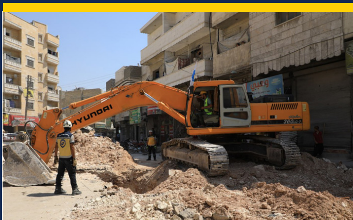
Rehabilitation of 3,300 meters of water networks and 5,050 meters of sewage systems in Al-Bab City.
